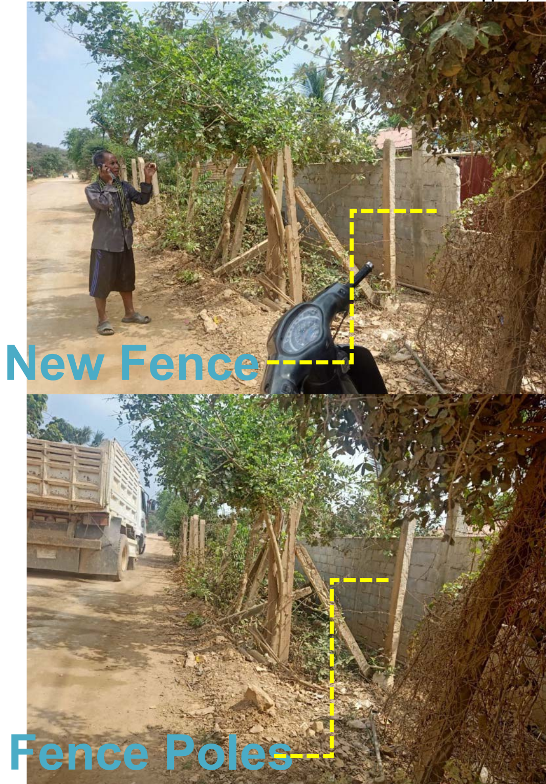
Photo 1: Front Fence Poles (Removable and mitigation was applied)
